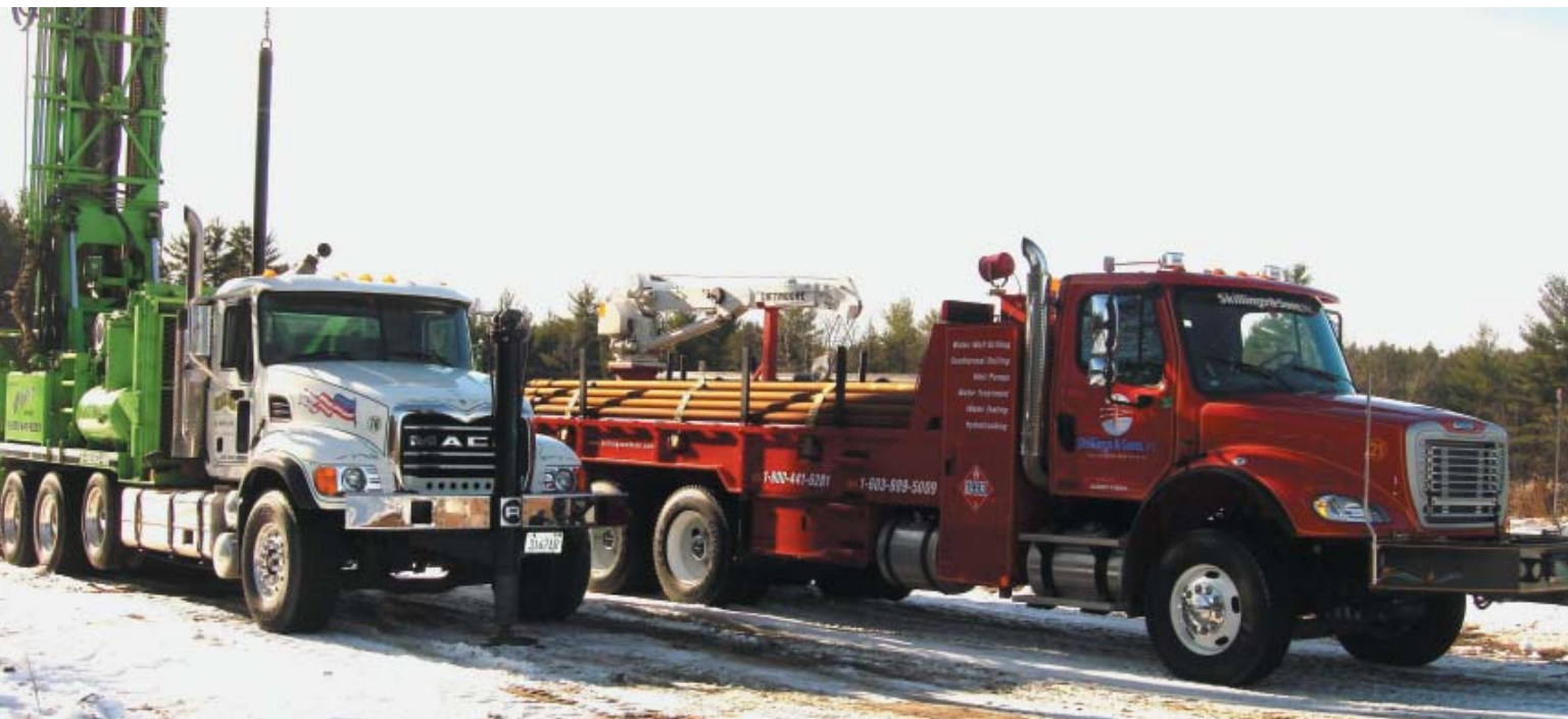
Specialized drilling equipment for use in the New England area can easily run into $800 thousand rigs to get through the geographic structures common in the area. Skillings has outfitted rigs for GSHP work to facilitate loop installation. (Photo courtesy of Skillings and Sons.)
