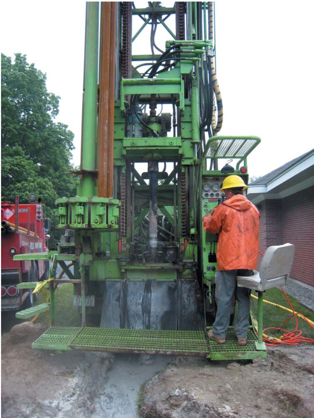
Roger Skillings stays actively involved in his drilling projects, and is as likely to man the rig as not. Skillings and Sons has the experience and equipment to do geothermal work in New England's demanding topography and is staying busy providing GSHP technology to commercial and residential clients trying to get ahead of the energy and expense increases expected this winter. (Photo courtesy of Skillings and Sons.)
